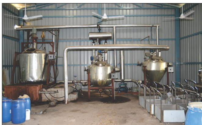
Machinery at Natural Dye Processing & Incubation Centre for Large scale paints production
